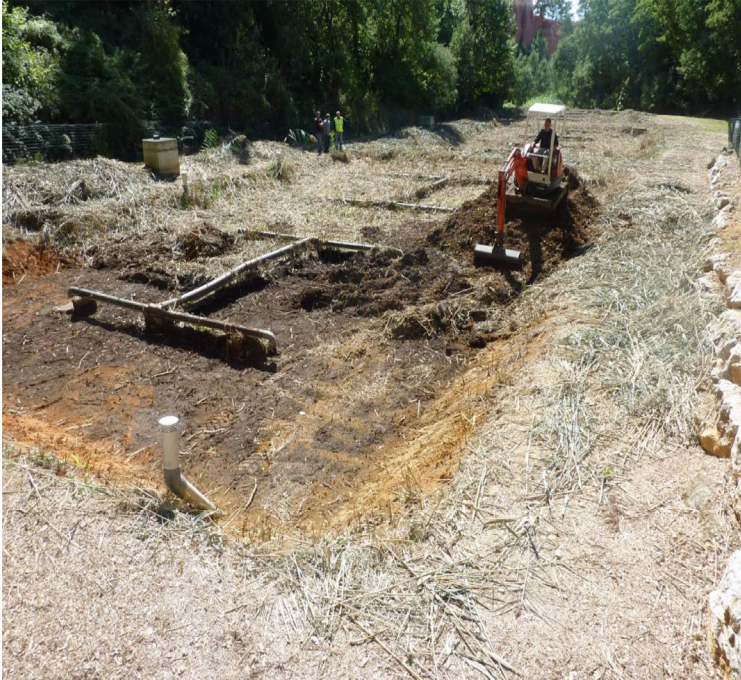
Figure 5.8 Sludge removal from the first stage French VF wetland in Roussillon, France after 13 years of operation (Troesch and Esser, 2012).
